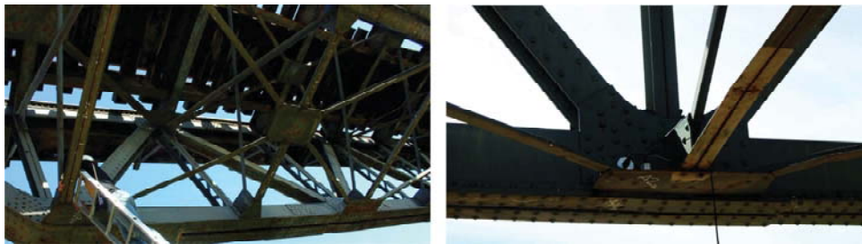
Figure 25: (left) Track in the Bridge over Jabalón River and (right) accelerometer at the truss connection.
