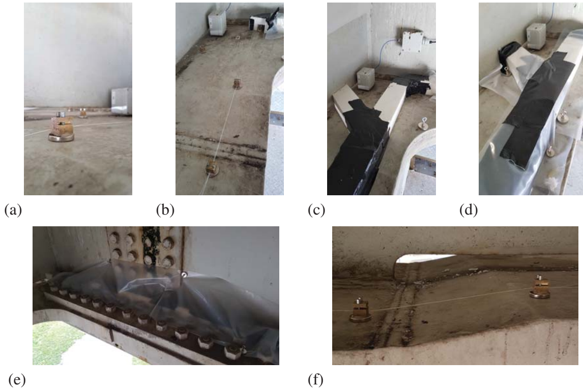
Figure 4: (a) and (b) Photo of mounted clamping blocks and glass fiber. (c) The thermal insulation, covering the clamping box and the fiber. (d) The plastic foil, covering the thermal insulation. (e) One of the steel connection plates. (f) The gap between a transverse beam and a girder.
