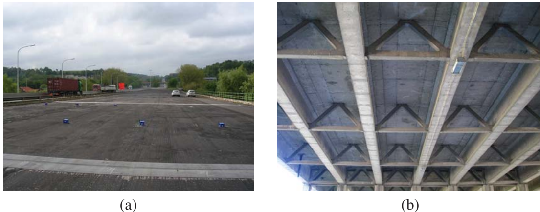
Figure 1: The Boirs viaduct, pictures taken during the tests: a) top view; b) bottom view.
