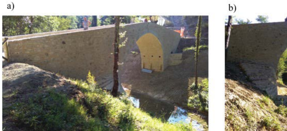
Figure 2: Images of the historic masonry arch bridge after the strengthening: general view of the South side (a) and wall (b).
